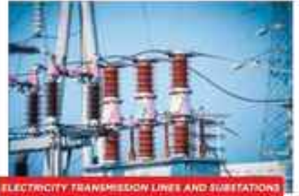
ELECTRICITY TRANSMISSION LINES AND SUBSTATIONS
